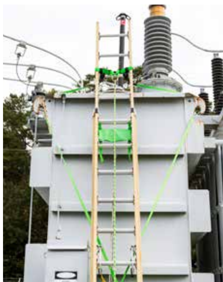
BLT attached behind lifting ears of transformer.
