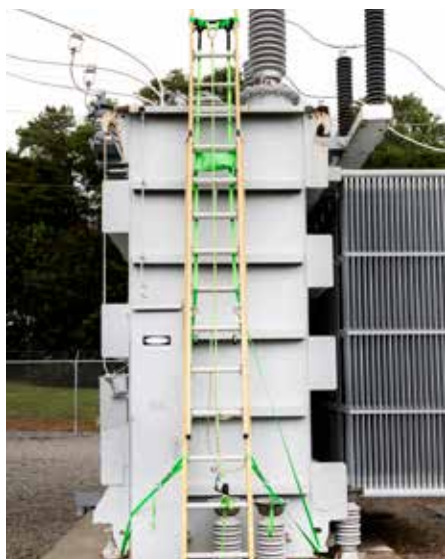
BLT attached to transformer (low mount).
