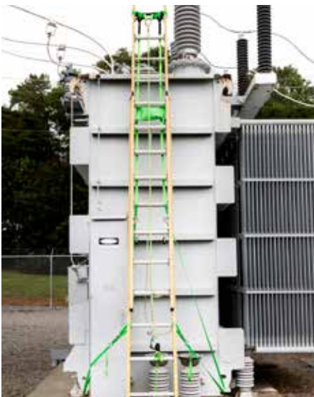
BLT attached to transformer (low mount).
