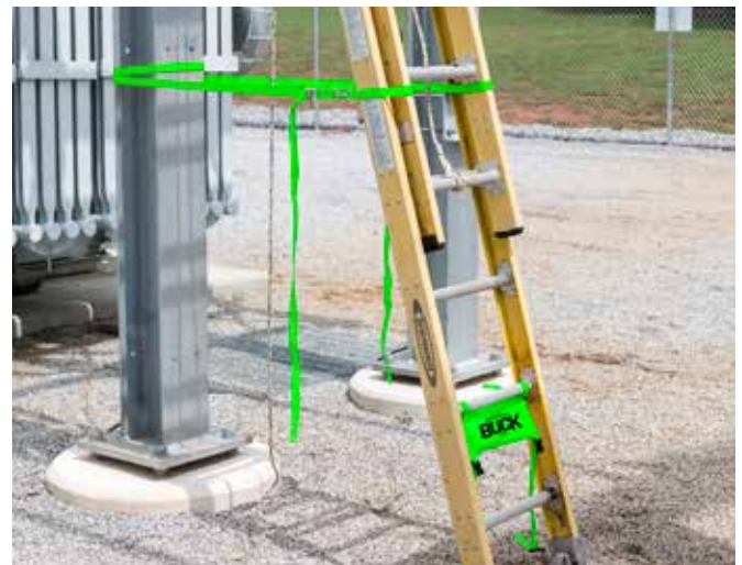
Ladder Lock (model 355B) used to secure ladder to steel prior to working.
