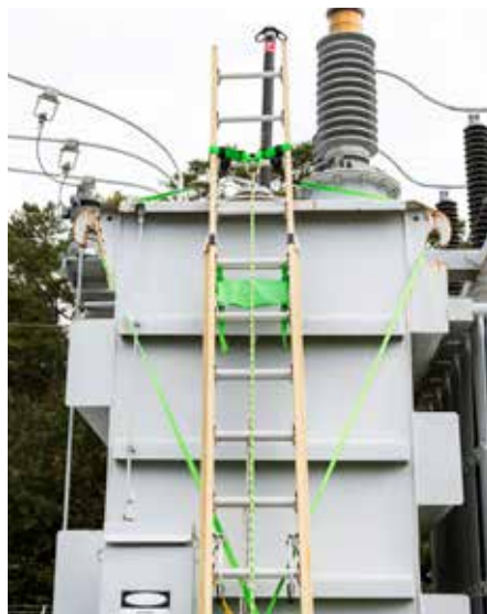
BLT attached behind lifting ears of transformer.
