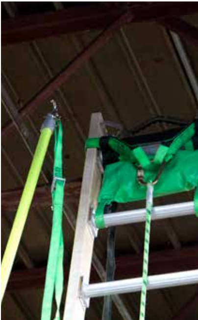
1. Once ladder is in place, use telopole to lift BLT straps over lattice.
