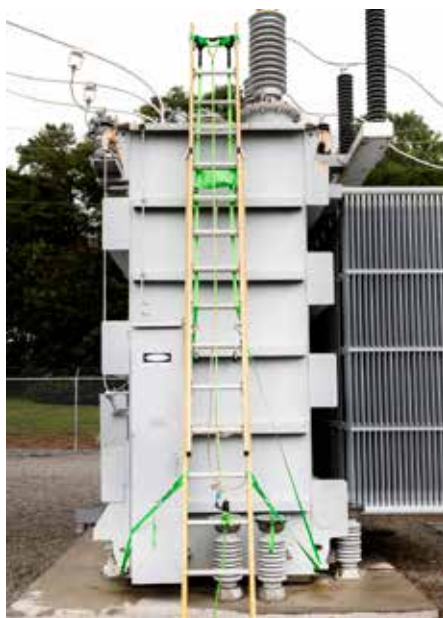
BLT attached to transformer (low mount) in a substation.
