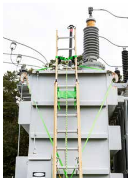
BLT attached behind lifting ears of transformer in a substation.
