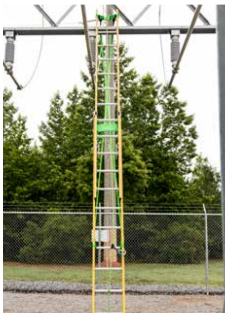
BLT attached to trussing in a substation.
